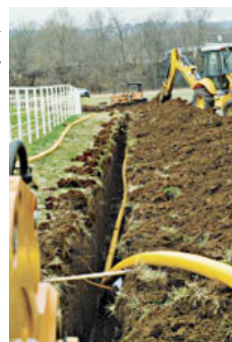
Arkema CALL BEFORE YOU DIG Polyamide 11 is used to make gas distribution pipes.
